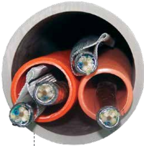
1" MaxCell overriding existing cable plant in a 3" duct
